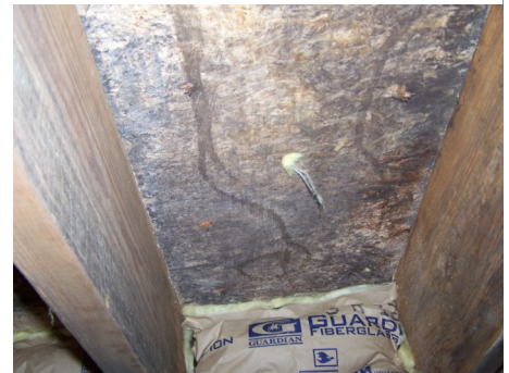
Picture of the contaminated crawl space.
