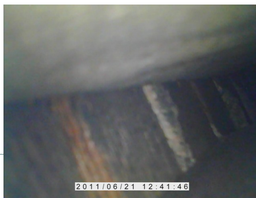
Soot inside the wall cavity.
