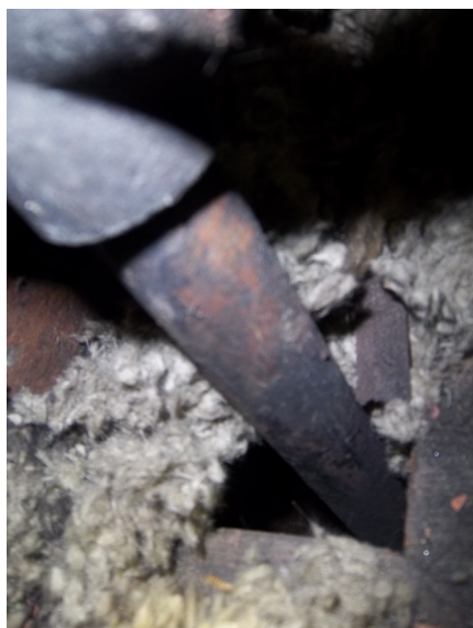
Picture of the oversized access hole. Notice the amount of soot around this hole.
