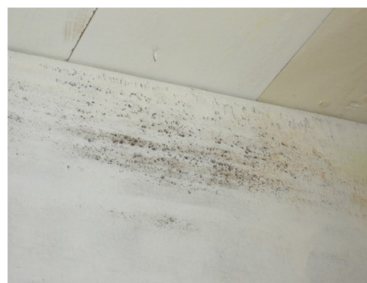
Mold growing through anti-microbial paint
